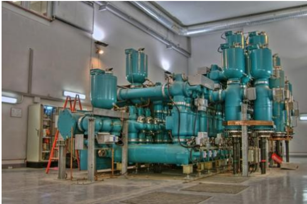
Gas Insulated Substation
